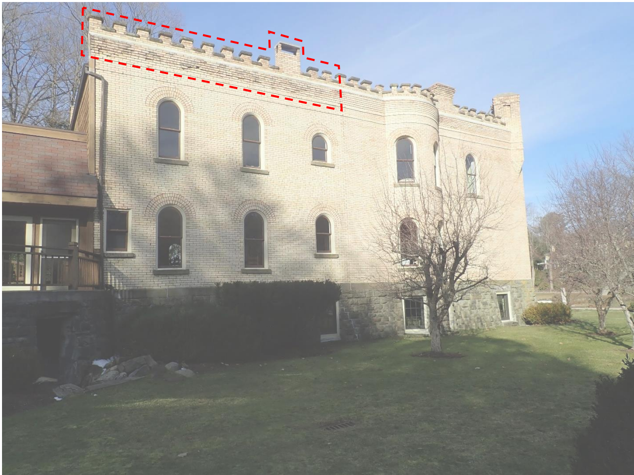
Figure 1. View of east facade, red box outlines the approximate extent of masonry to be repaired per our understanding of the project scope.
